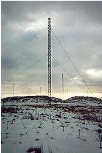
One of the many rusting tower farms on Shemya Island. The sky bears witness to Bering Sea and Pacific Ocean storm fronts moving in.
